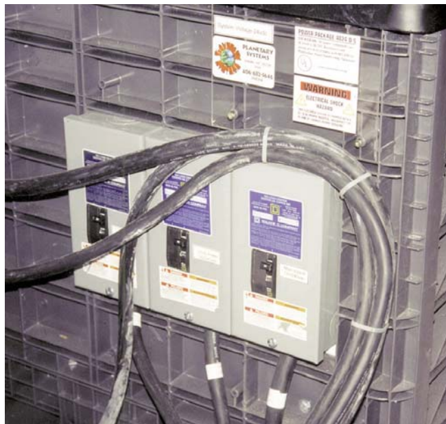
Generator, utility power, and main output breakers.
