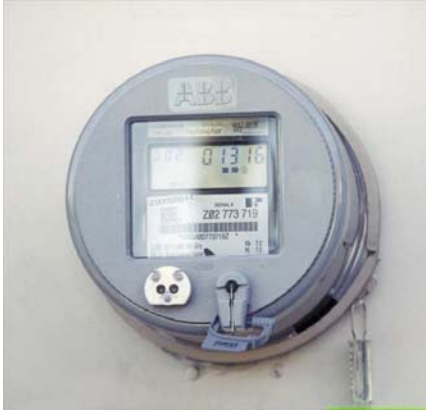
The utility meter records both incoming and outgoing kilowatt-hours.
