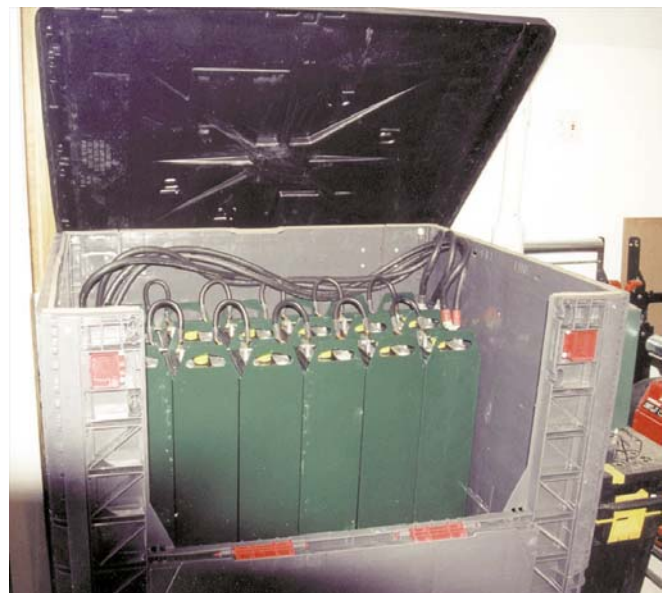
The battery module provides vented containment for the twelve IBE lead-acid cells.
