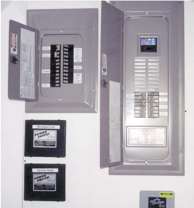
The main grid panel and subpanel with the automatic transfer switches for the ovens, below.
