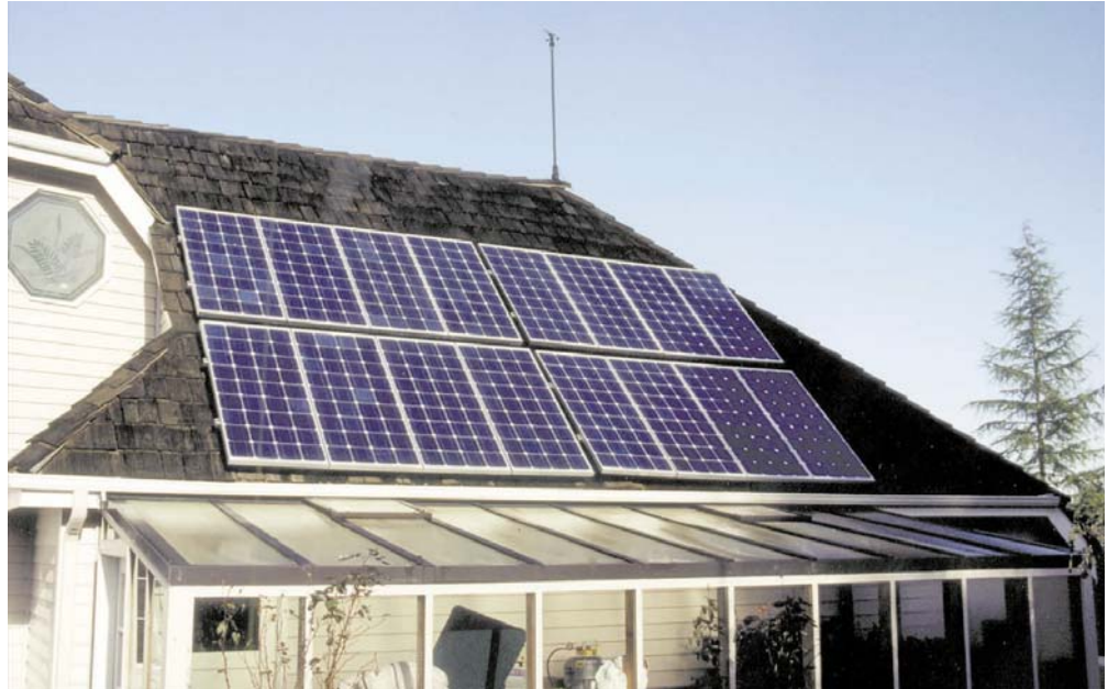
Sixteen AstroPower PV modules, for a total of 1,920 rated watts, are mounted on the south-facing roof above the greenhouse.
