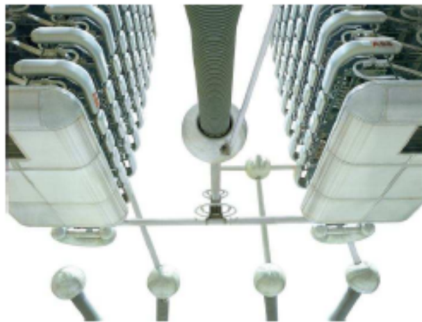
Figure 25.13: A high-voltage DC power system in China. Photo: ABB.
