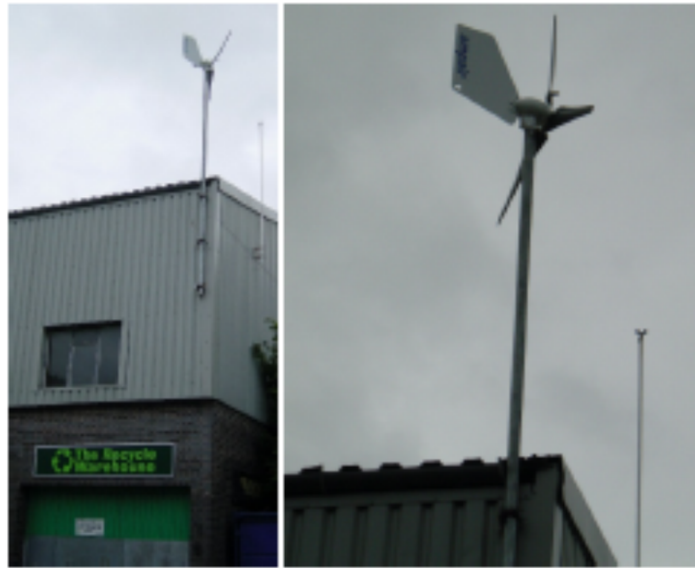
Figure 14: Bad: An Ampair “600W” micro-turbine. The average power generated by this micro-turbine in Leamington Spa is 0.037 kWh per day (1.5W).
