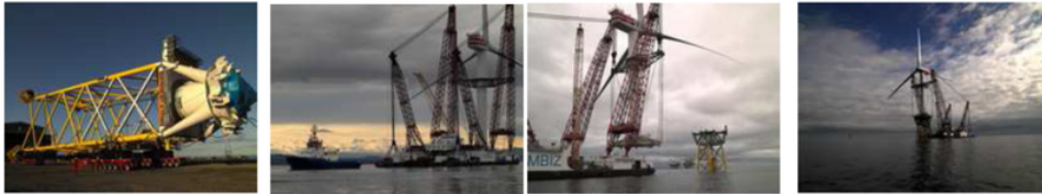
Figure 10.8: Construction of the Beatrice demonstrator deep offshore windfarm. Photos kindly provided by Talisman Energy (UK) Limited.
